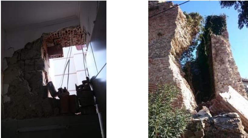
Fig. 17. Crushing failure of the walls
