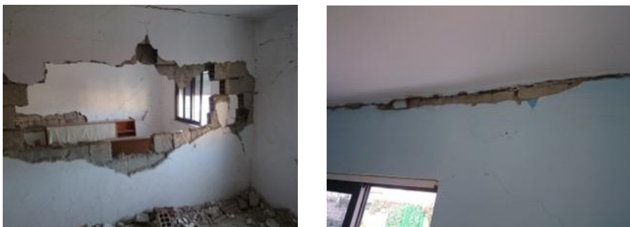
Fig. 10. Observed out-of-plane collapses of walls
