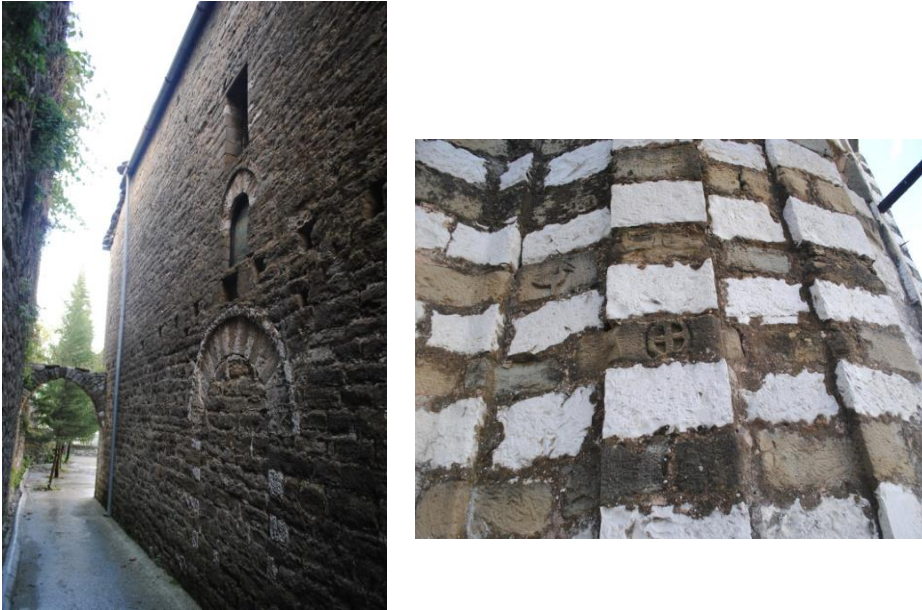
Figure 4. Western wall of the Basilica (left); Different colored stones, Eastern wall of the Basilica (right)
