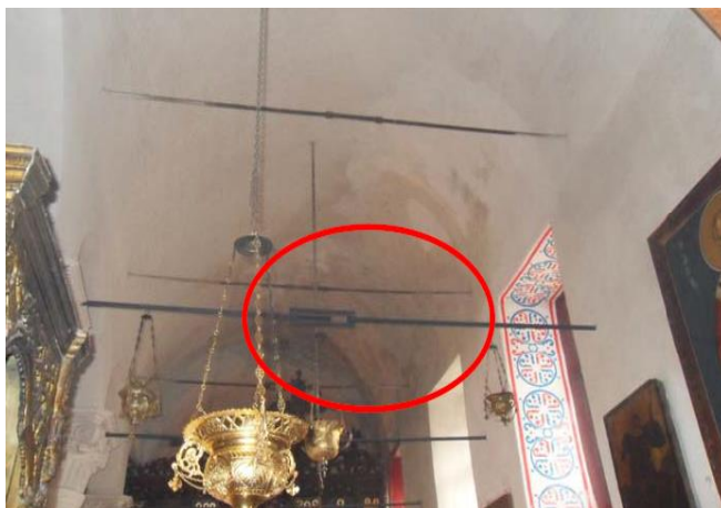
Figure 6. Barrel vault over the South aisle, moisture concentration
