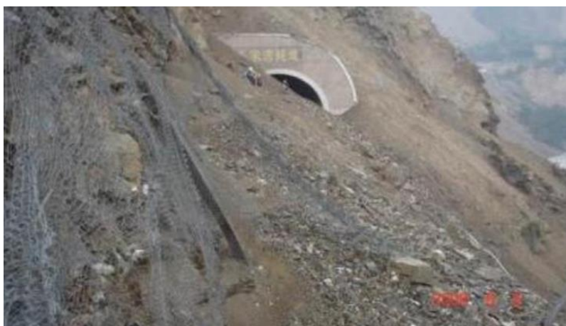
Fig. 3 Tunnel portal failure due to slope instability after Chi-Chi earthquake(28)
