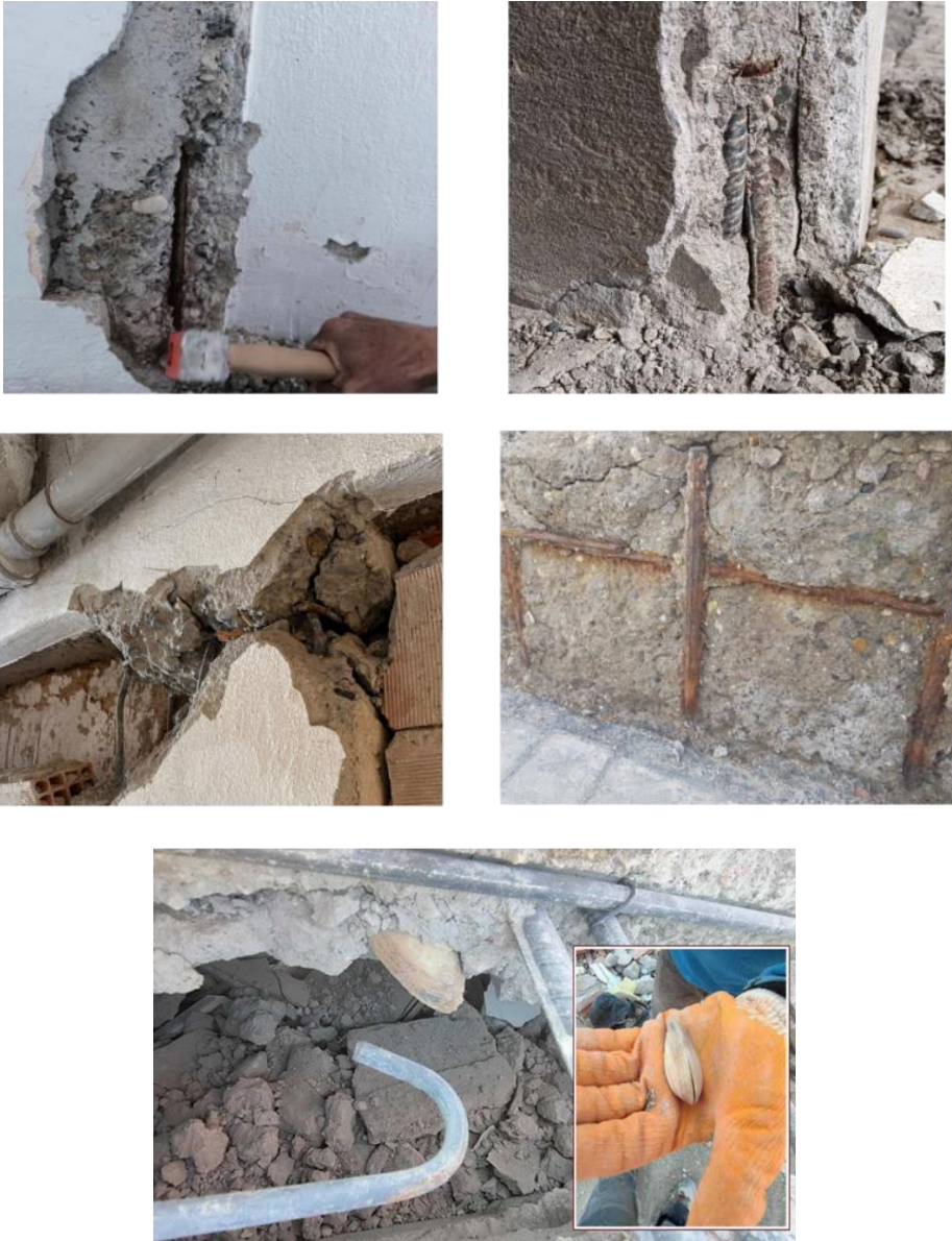
Fig. 1 On-site images of corrosion formation in earthquake site, Turkey
