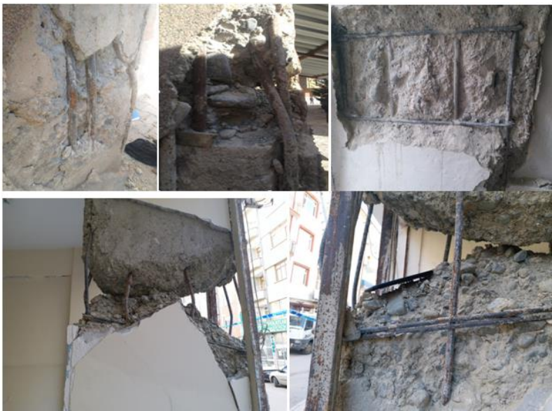
Fig. 3 Damages in RC according to poor/low strength after 2020 Sivrice earthquake
