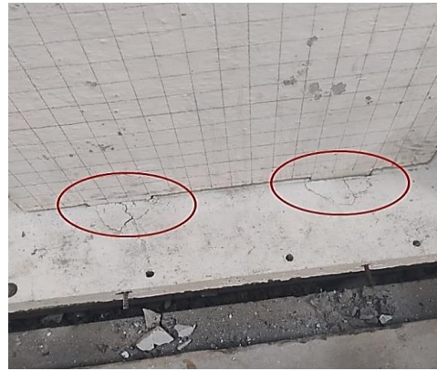
Fig. 15 Initial failure of RW joints with connector
