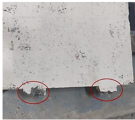
Fig. 12 Failure from RW1 specimen
