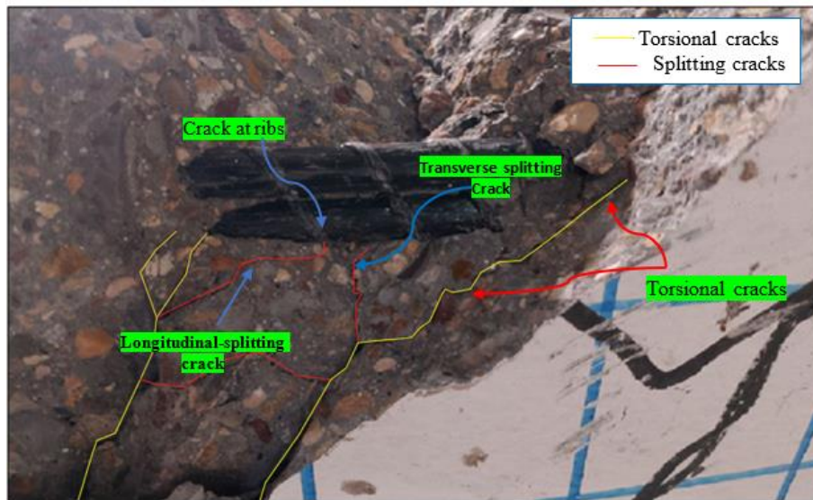
Fig. 13. Cracks types within splice region(G-Lap300)
