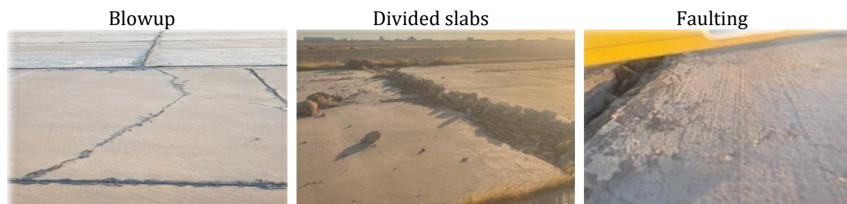
Fig. 5. Concrete pavement distresses
