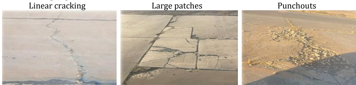
Fig. 6. Types of cracks and patches in runway slab
