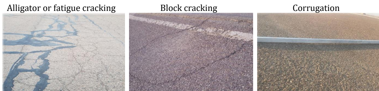
Fig. 2. Asphalt pavements distresses
