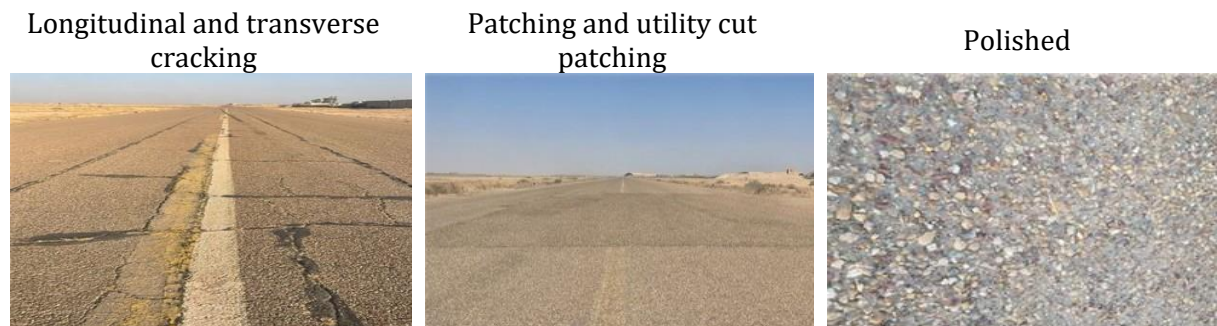
Fig. 3. Problems of asphalt runways
