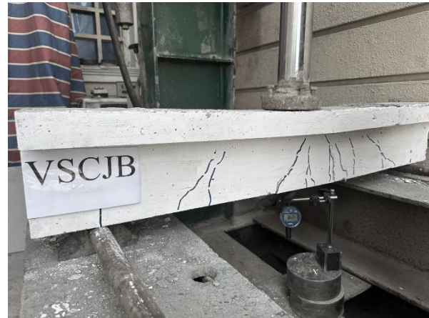
(b) vertical joint in shear span (VSCJB)
