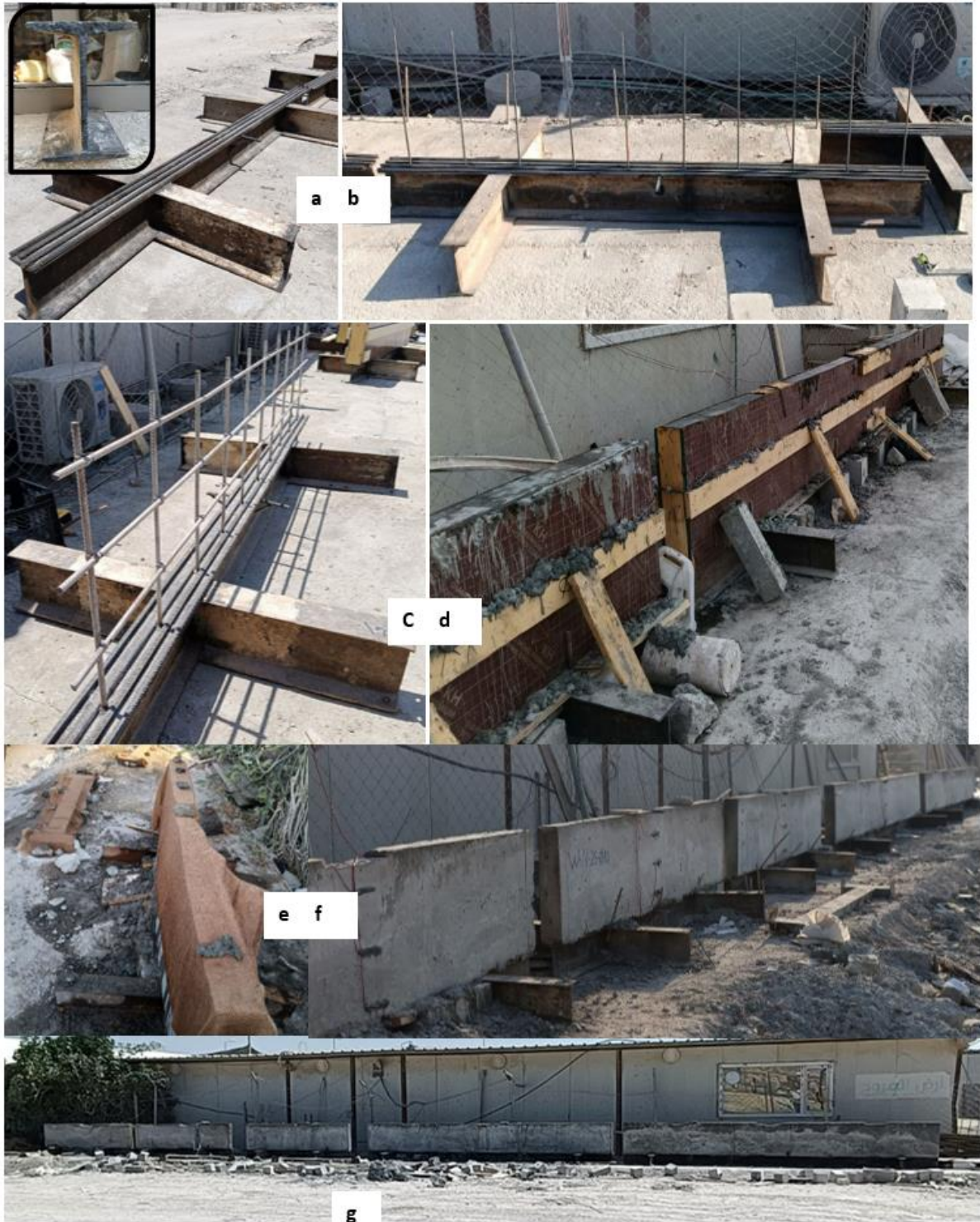
Fig. 2. (a), (b), (c) preparing walls, (d) casting, (e) curing, (f) strain installation., (g) The five hardened walls
