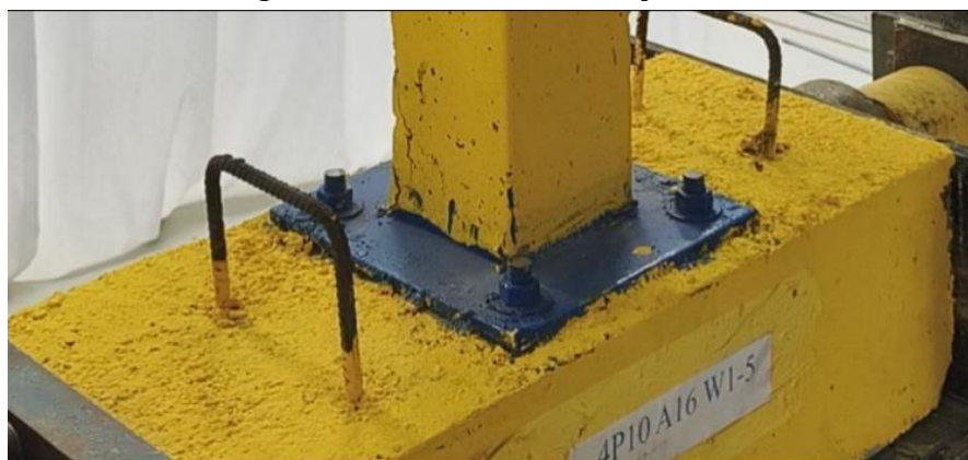
Fig. 20. Failure mode of (4 P10 A16 W1 -5) specimen
