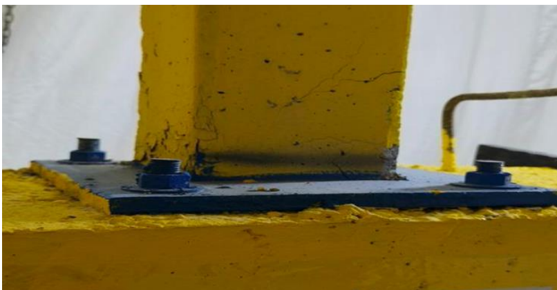
Fig. 23. Failure mode of (4 P15 A16 S -4) specimen
