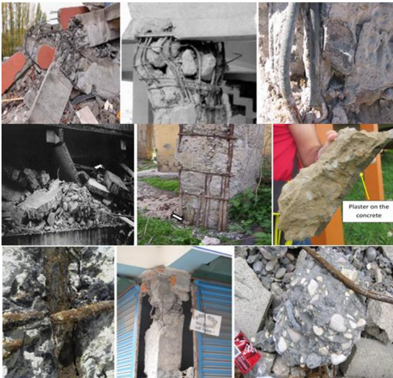
Fig. 4 Poor quality/ low strength material damages after different earthquakes [29-37]
