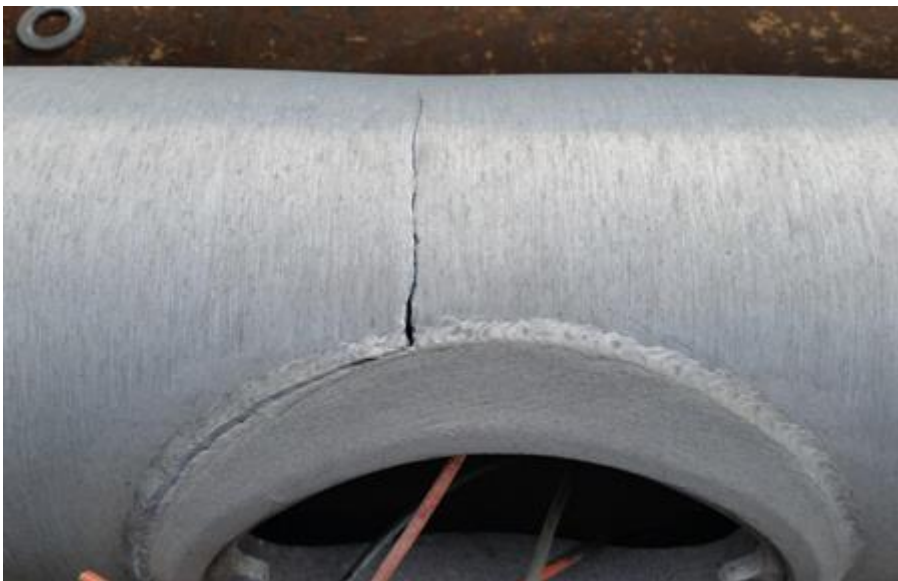
Fig. 1 Fatigue crack in welded aluminum light pole hand-hole in field
