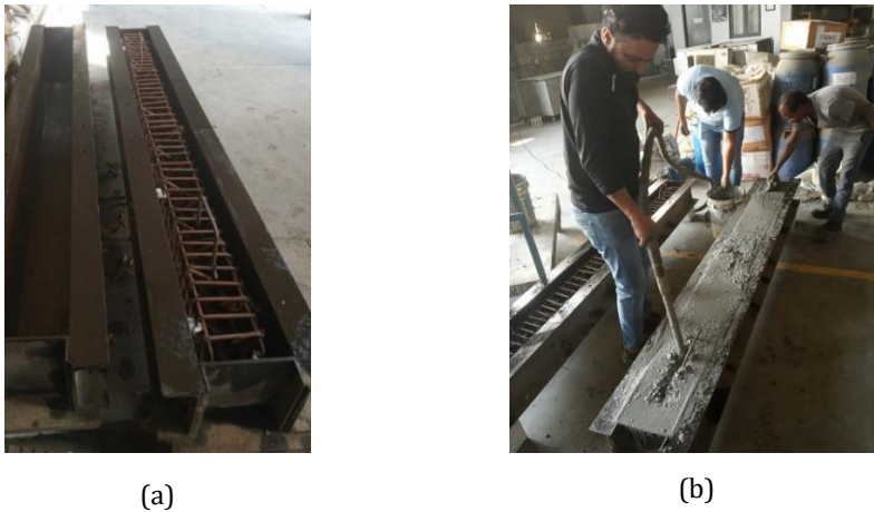
Fig. 2 (a) Reinforcement and mould for preparing the specimen and (b) Casting of specimen
