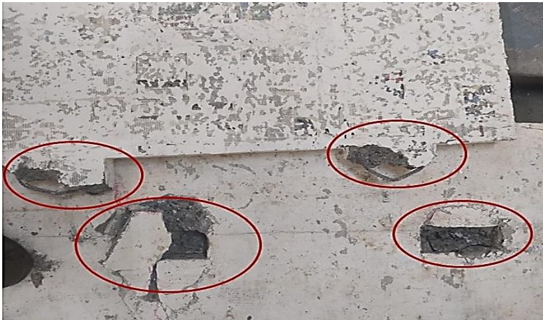
Fig. 16 Complete failure of RW joints with connector
