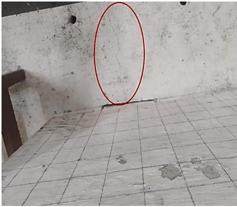
Fig. 14 Shear crack from the specimen with connector
