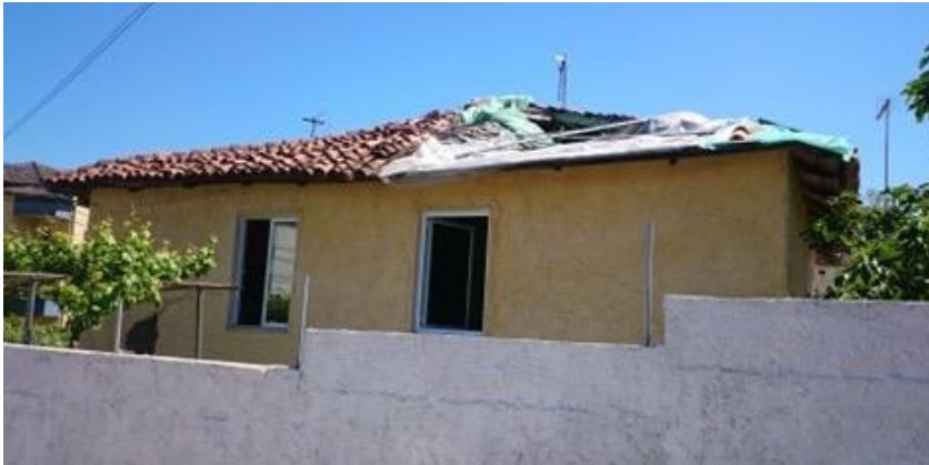
Fig. 6. Collapse of masonry buildings
