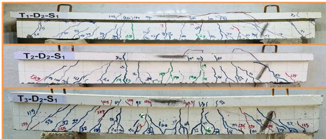
Fig. 12. Crack patterns and failure modes for T-beams reinforced with steel bar of 12 mm
