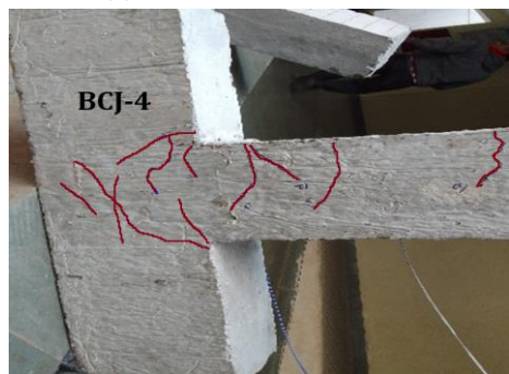
(a) Crack Patterns of BCJ-4
