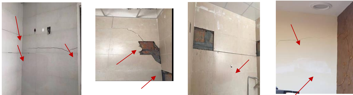
Fig. 2. Shape and position disparate fissures in the examined residential compound in Kirkuk, Iraq
