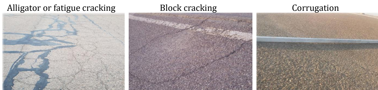
Fig. 2. Asphalt pavements distresses
