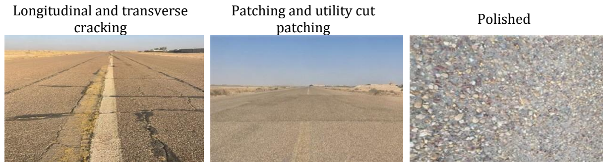
Fig. 3. Problems of asphalt runways
