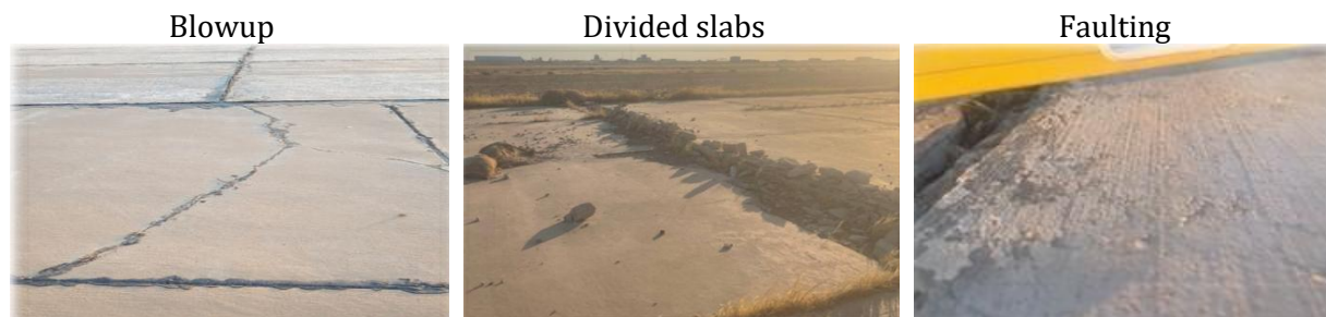
Fig. 5. Concrete pavement distresses
