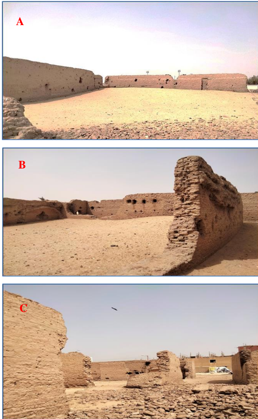
Fig. 8. A. and B. the courtyard of the citadel. C. the destroyed architectural units of the citadel
