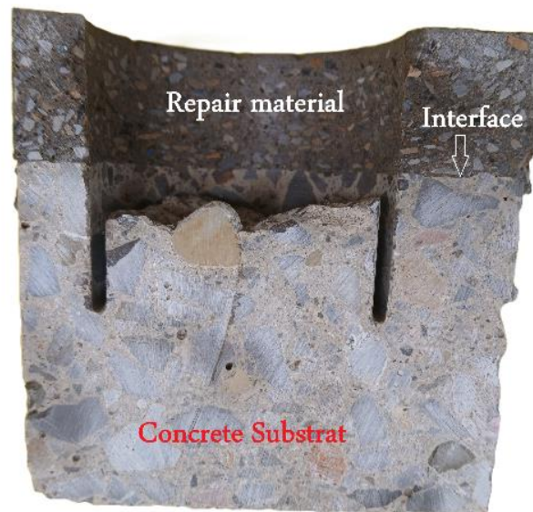
Fig. 10. Failure modes of SCSC-repaired specimens
