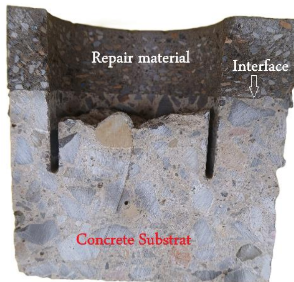
Fig. 10. Failure modes of SCSC-repaired specimens
