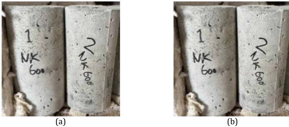
Fig. 11. Physical condition of normal concrete specimens before and after exposure to 600°C: (a) before burning, bright gray in color; (b) after burning, showing no significant color change, with increased localized yellowish spots, longer cracks, and spalling
