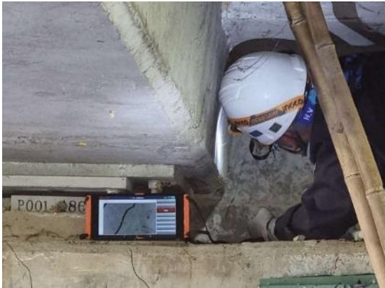
(a) Measurement of surface crack width using ZBL-F130
