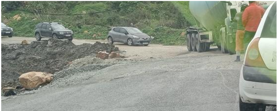
Fig. 1. Example of pavement instability in the Tizirt region
