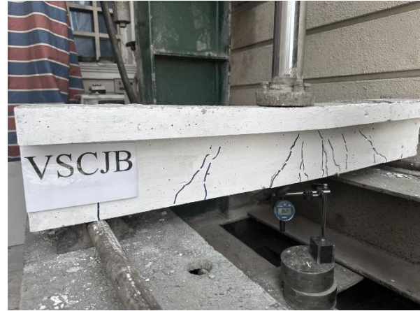
(b) vertical joint in shear span (VSCJB)
